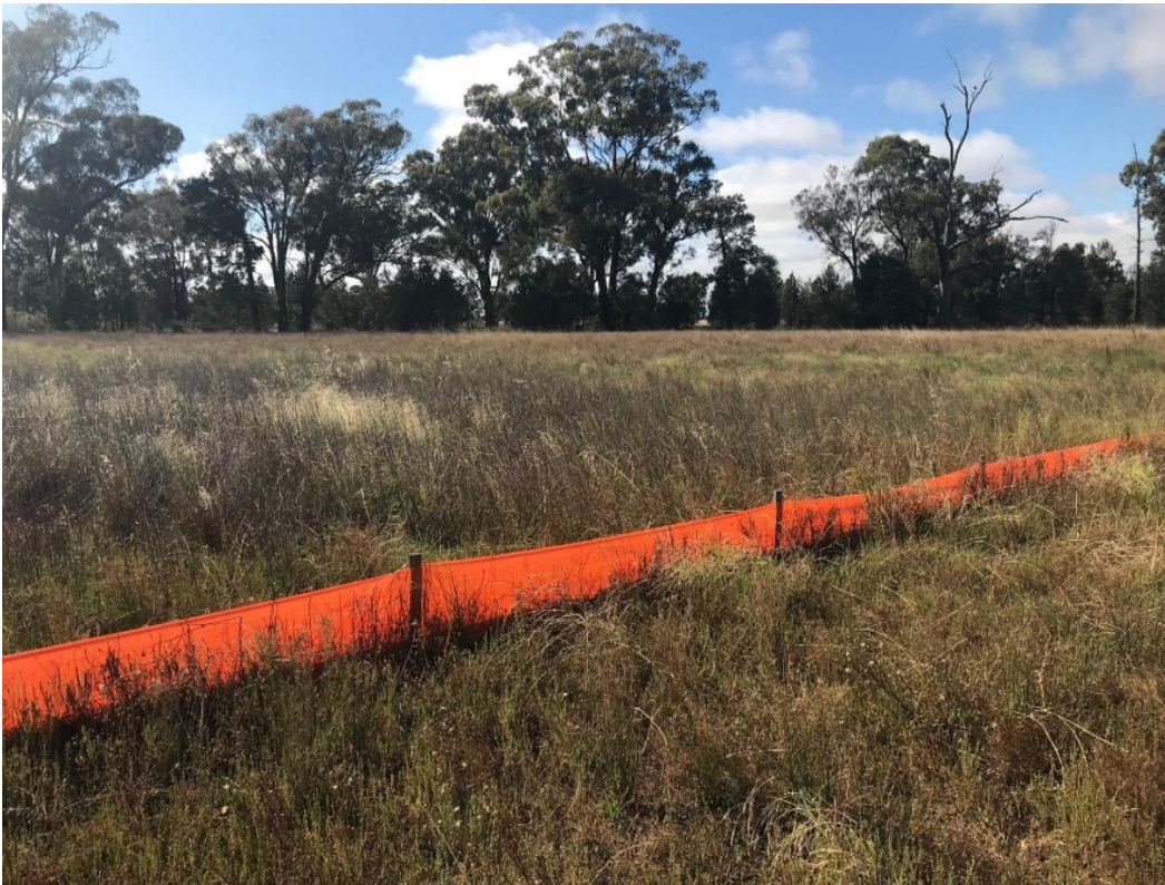
Photograph C.11 Sediment fences had been re-established after the flooding
