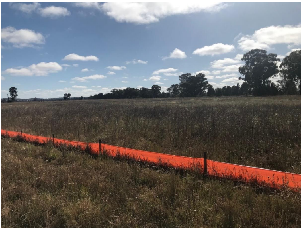
Photograph C.12 Sediment fence along boundary line
